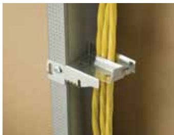
Metal Stud with non-metallic sheathed cables
